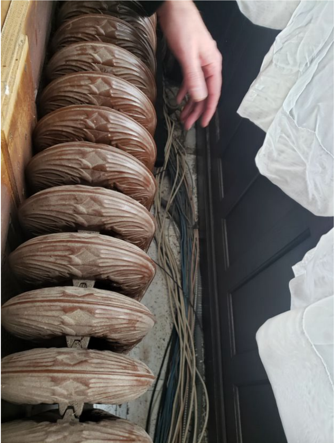
Figure 5: Cable Installations Near Radiators - Typical
