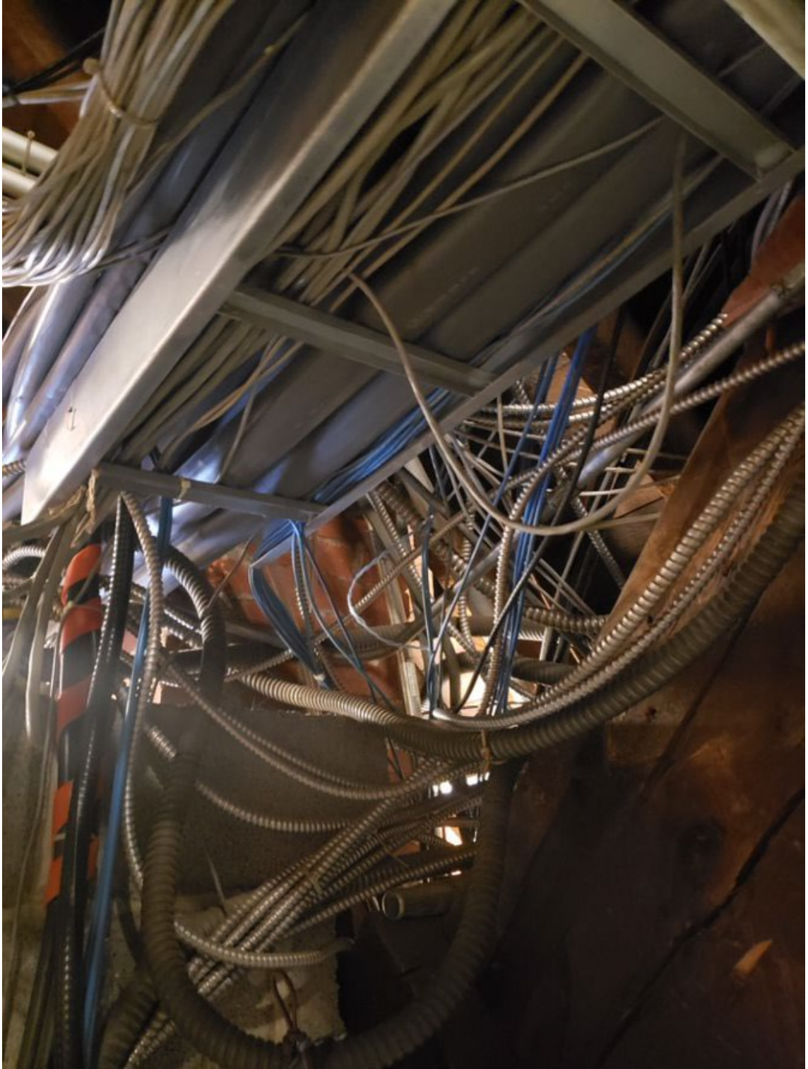
Figure 1: Cable Trays Filled Beyond Capacity - Typical
