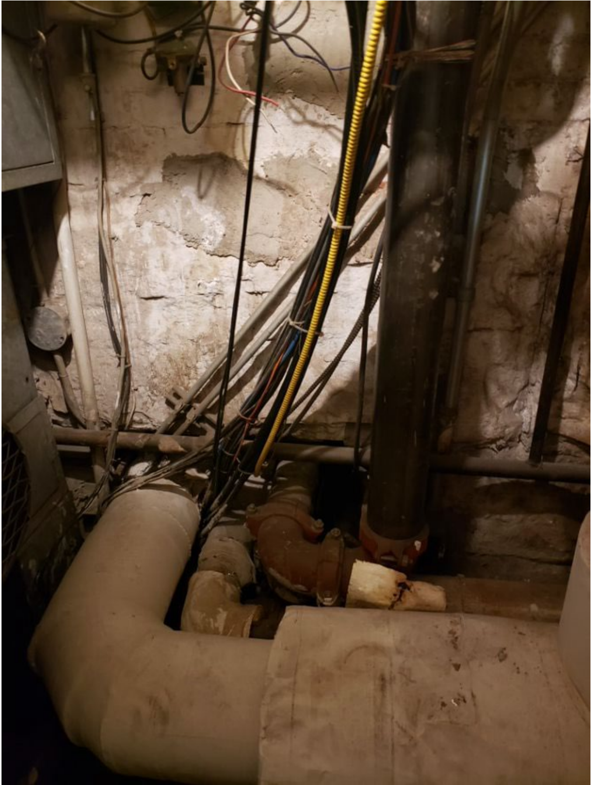
Figure 10: Original Main Steam Supply to the Legislative Building
