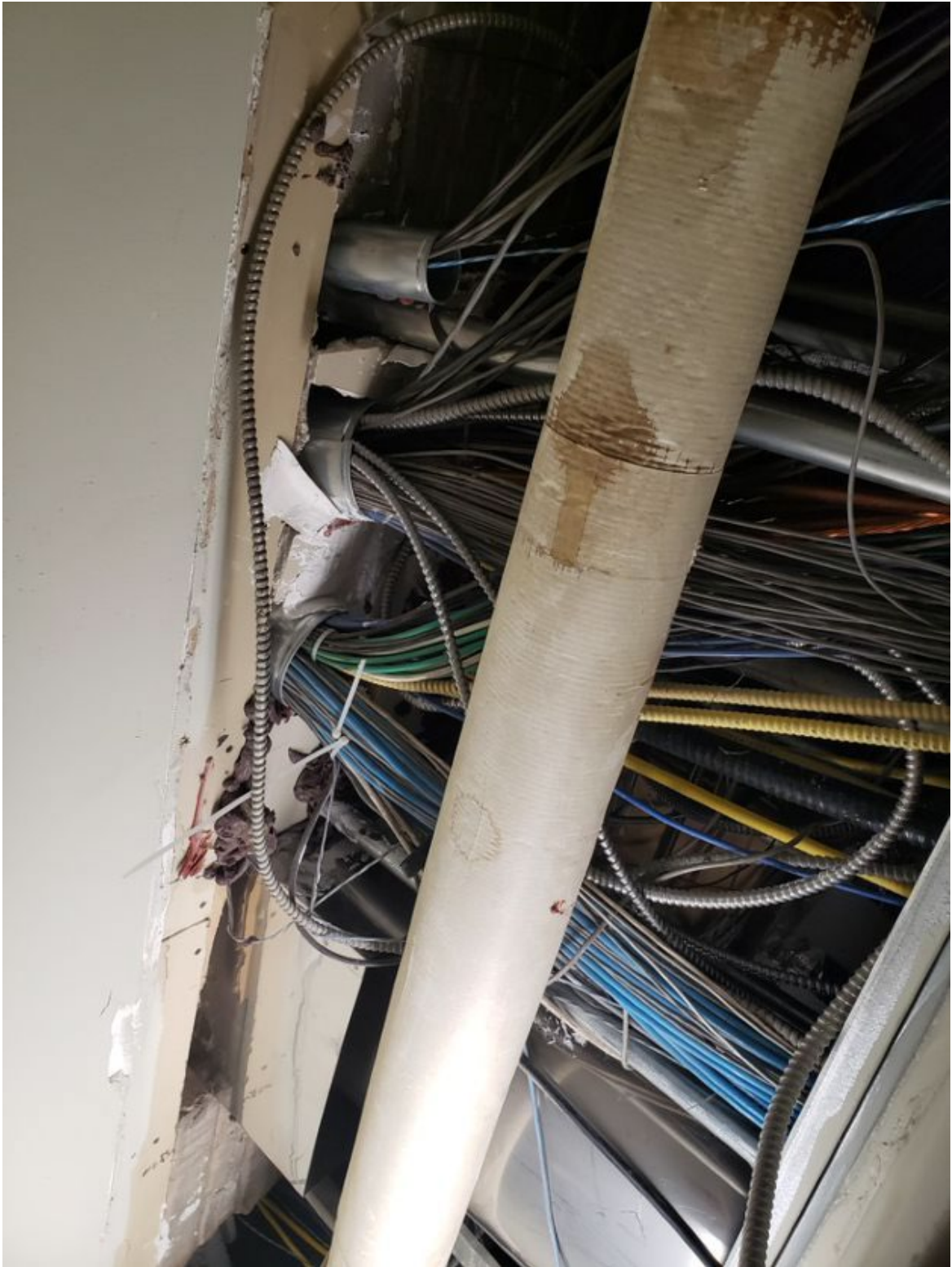
Figure 7: Masonry Shaft, Disorganized and Unidentifiable Cables throughout Shaft and Ceiling Spaces throughout Basement
