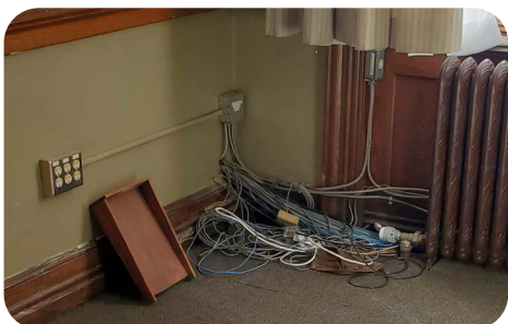
Exposed wiring in an office. Insufficient power and outlet locations and lack of cable distribution pathways have led to an overabundance of wiring in offices.
