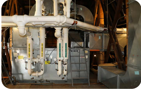
Current HVAC units in the attic. They are close to the end of their lifecycle and need to be replaced.
