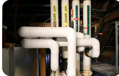
Steam pipes in the attic. Steam heat is inefficient and problematic in the summer months. Steam heated radiators overheat the building during the winter months.
